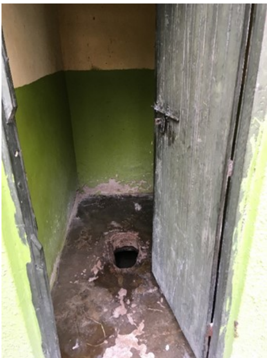
Inadequate menstrual hygiene pit at Muko High School
